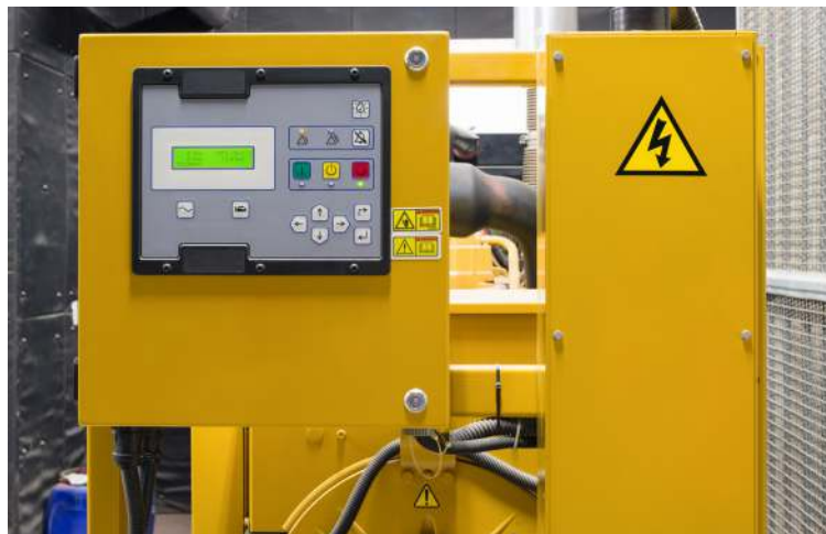
Figure 7: Typical UPS Monitoring
